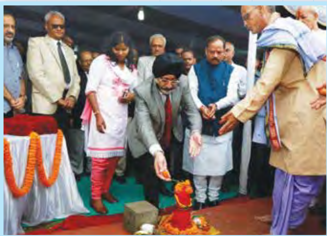
Commencement of Construction Work of New Building of High Court of Jharkhand at Dhurwa, Ranchi
